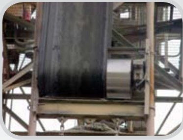
A typical mistracking problem resulting in product spillage and possible damage to the belt, mechanical splices and/or conveyor structure.
